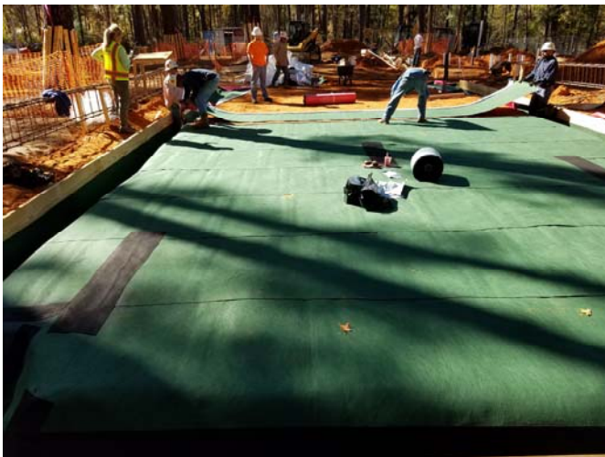
TERM Underslab Barrier – Visitors Center – Mission TX
