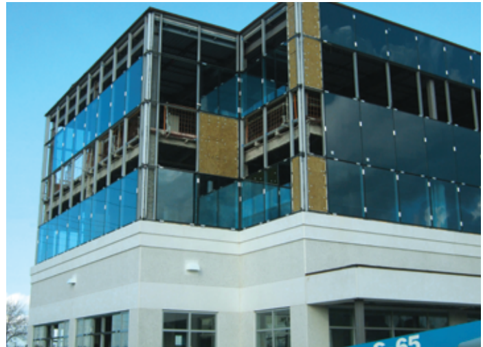
Developer Monterey Park used ROCKWOOL CURTAINROCK® insulation for its recently opened 75,000 sq. ft. commercial building in Brampton, Ontario.
